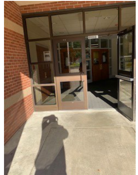
Propping doors open is a no no!
